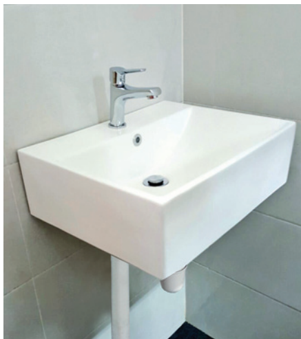
Wash basin with tap mixer
